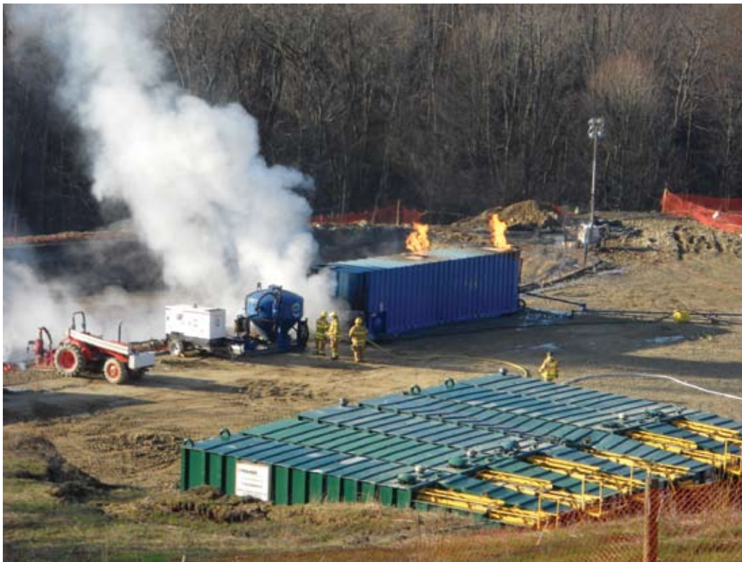
Volunteer firefighters respond to a fire in a wastewater pit at an Atlas Energy Resources well site in Washington County, Pa., in March 2010. Fracking places increased demands on emergency responders, creating new dangers that require additional training, and increasing demands for response to traffic accidents involving heavy trucks. Credit: Robert Donnan
