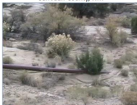
Exposed Gathering Pipeline San Juan County, NM
